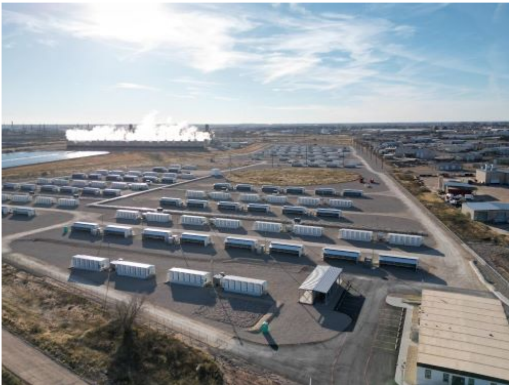
Odessa Data Center Area B & C
