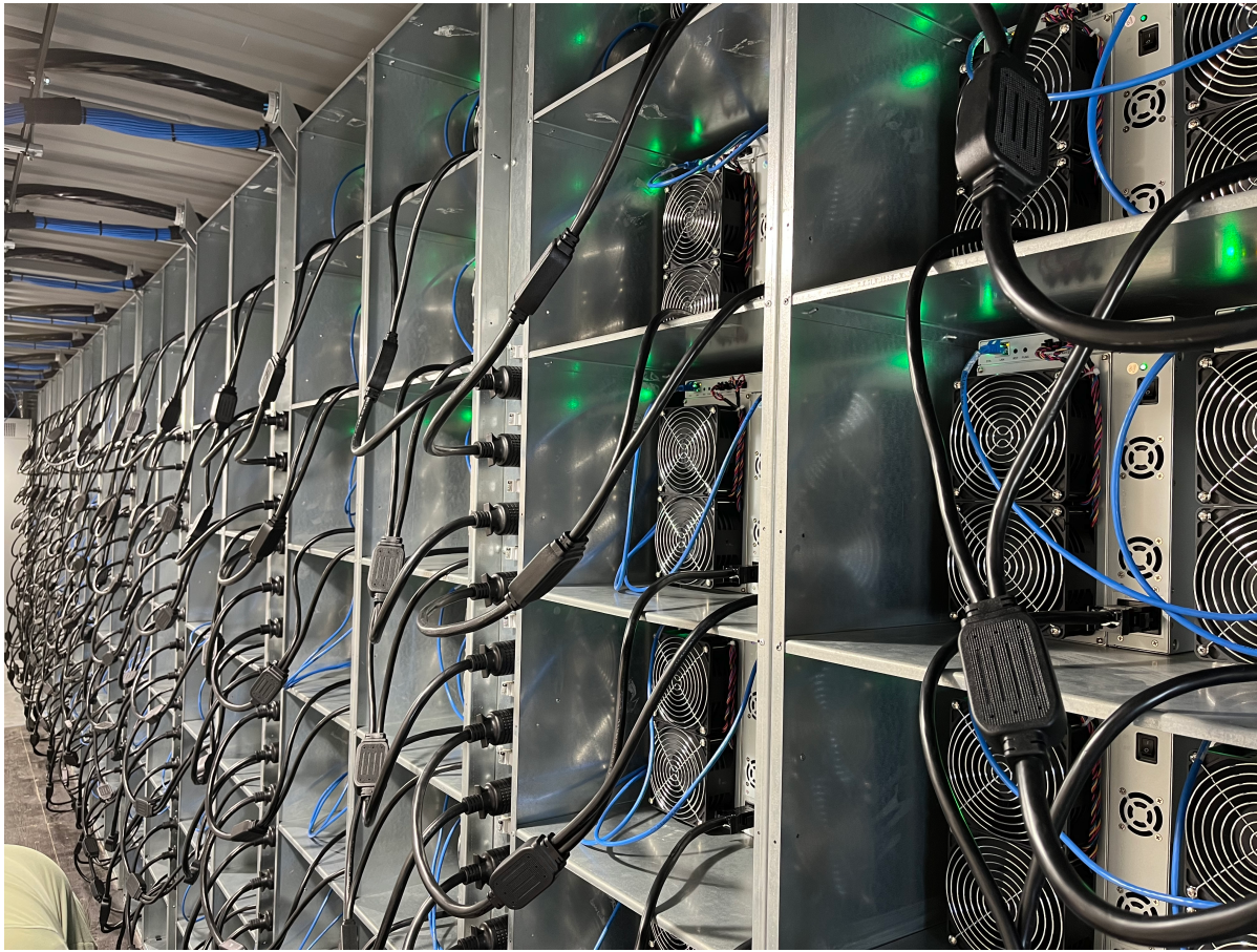
Recently Installed Canaan Rigs
