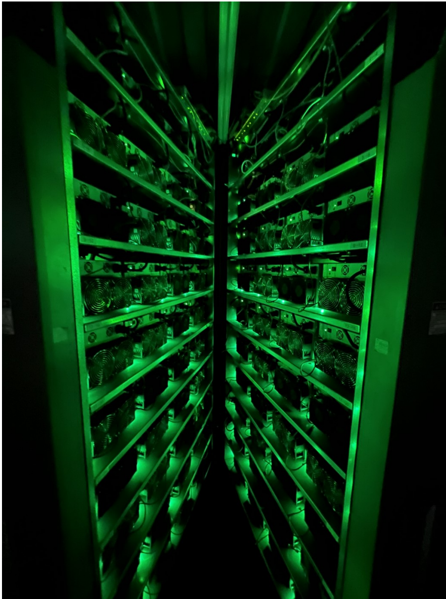
Cipher Mining's Rigs at the Odessa Data Center
