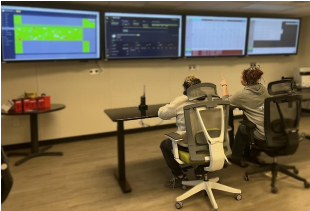
Operations Center at Cipher Mining's Odessa Facility
