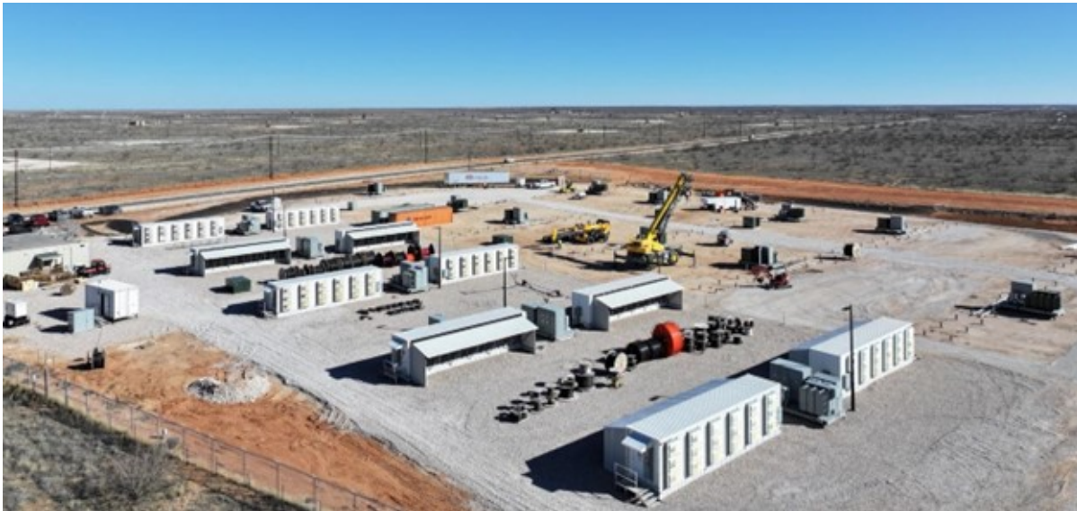
Bear 30 MW expansion on track for Q2 2024 energization
