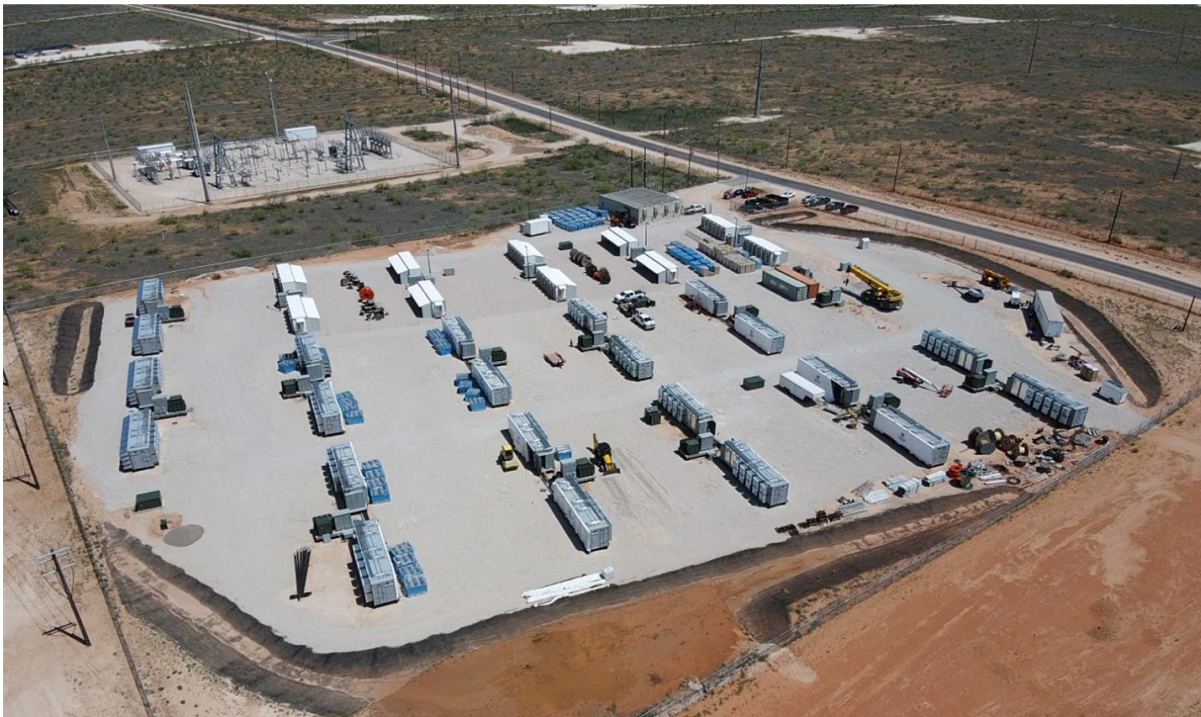
Completed infrastructure at Bear with 30 MW expansion on track for Q2 2024 energization
