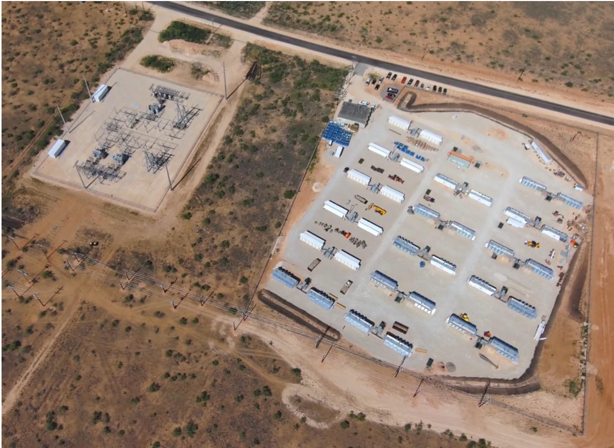
30 MW expansion at Bear is energized and ramping hash rate
